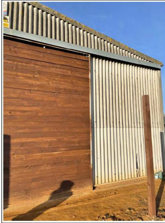
Photo 3 (taken from Anthony-Johnson Consulting Engineer Ltd. report): Part of the eastern aspect of the barn, showing the existing barn doors.
